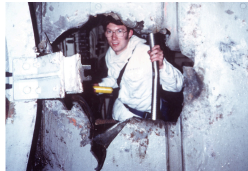
Lt White inspecting the bomb damage
